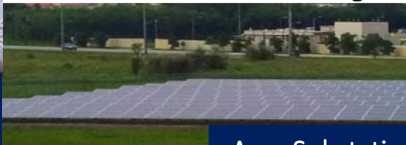
Apra Substation Site
